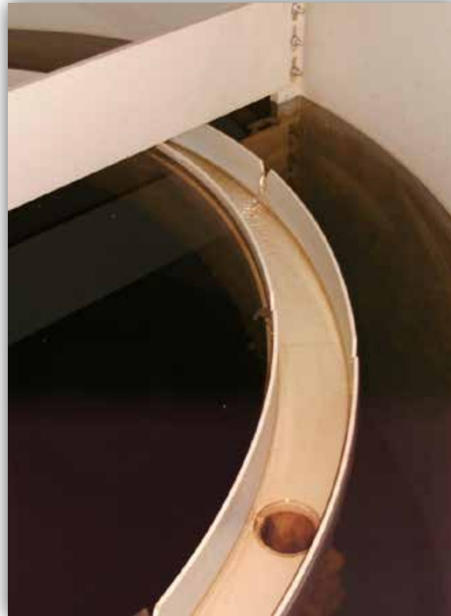
Effluent of secondary clarifier
